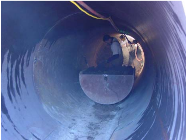
Tunnel being built under the railroad tracks at Allen Park to accommodate the new Allen Park interceptor
