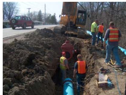
Water main extended to Heritage Harbor (corner of Old Chicago Road and Canal Road)
