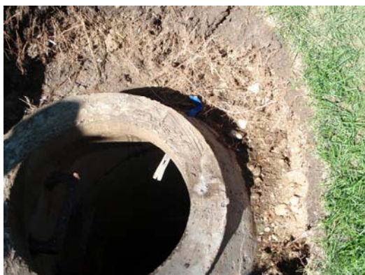
Manhole defect (see pry bar in the manhole allowing storm water into sanitary sewer system)
