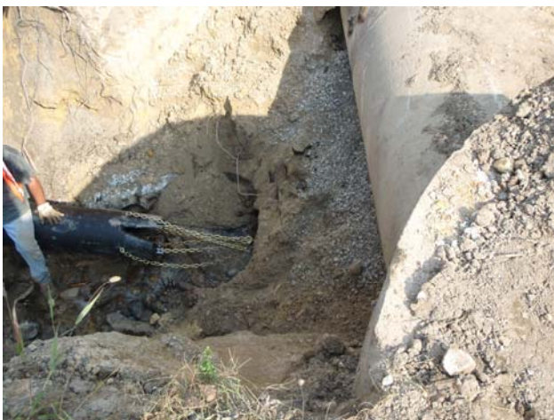
150 feet of high density polyethylene (HDPE) pipe was pushed through the existing sewer under Route 71 by Larry's Universal to avoid digging up and closing Route 71. Third Avenue sewer (Center Street to Van Buren) was also relined by Larry's Universal
